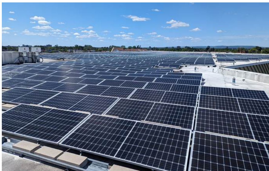
Photovoltaic panels on the roof of the Student Commons
