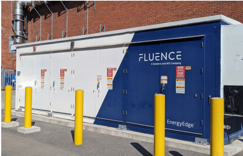
Figure 2 Battery Storage System
